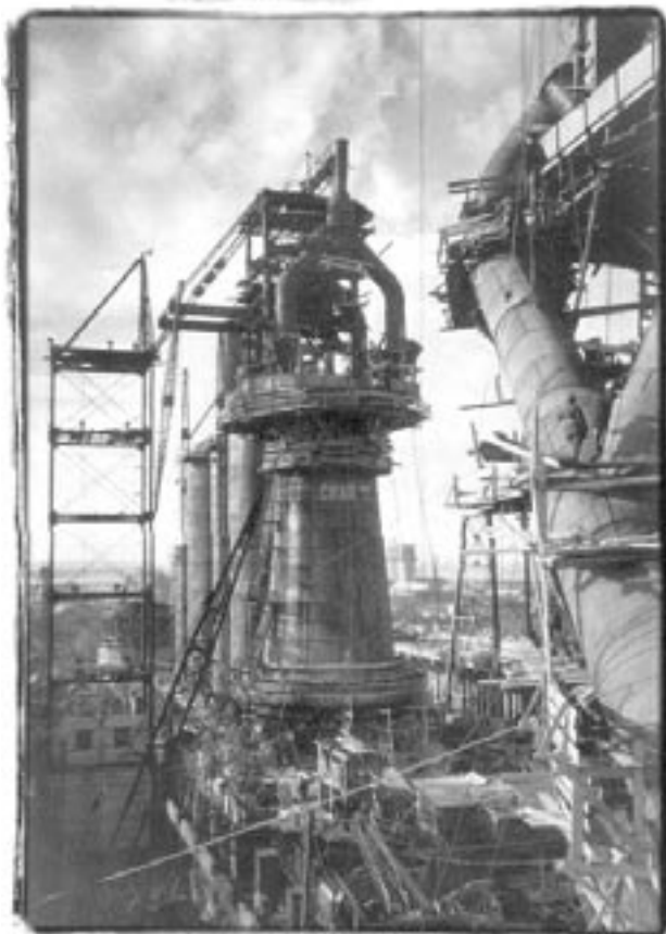
On her second trip to the Soviet Union, Margaret photographed a blast furnace under construction in Magnitogorsk.
